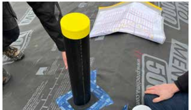
... and sealing of a vent pipe using the ROFLEX variant for pipe diameters of 100 - 120 mm (4" - 4 3/4").
