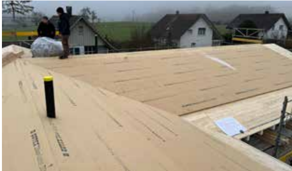
Positioning of the prepared sheet package for installation over wood-fibre underlay panels
